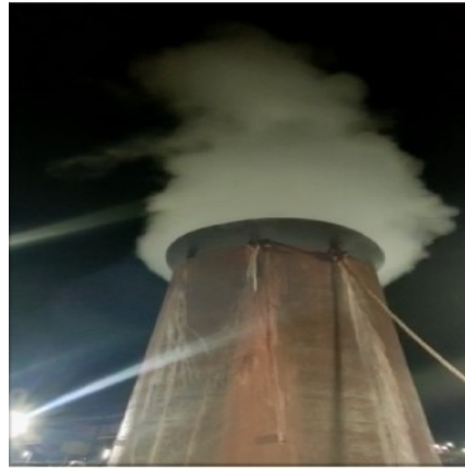
Figure 2. Vapor from relief tank.
